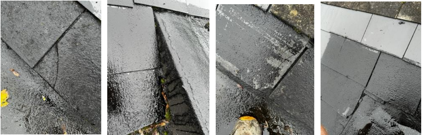
south east facing incorrect fixings and out of bond slates
