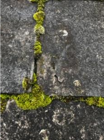
South west facing warn out slates
