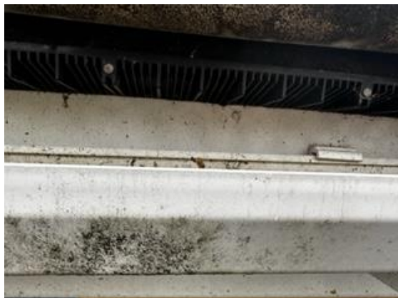
Incorrect fascia vent
