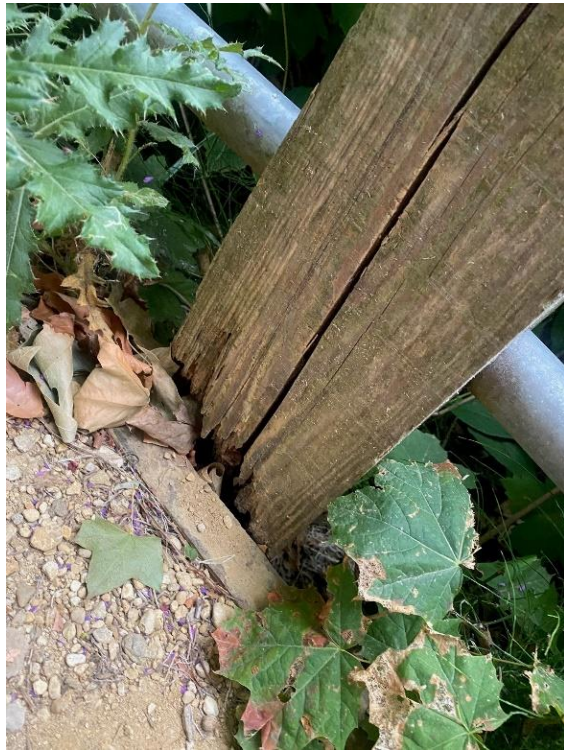
Wooden fencing supports now rotting
